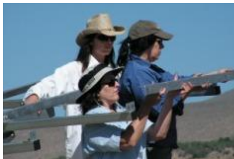
Women assemble a rack for a solar PV system at SEI's Paonia, CO eco-campus. © Solar Energy International
